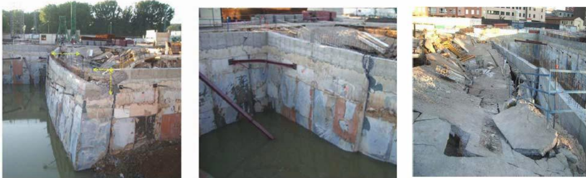
Figure 1 collapse of the stretch of wall screen.
