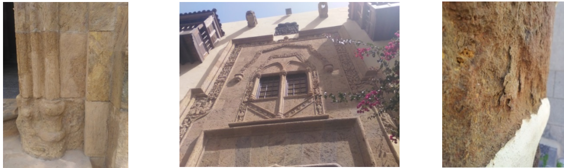
Figure 1 Materials degradation at Colón's house in Vegueta.
