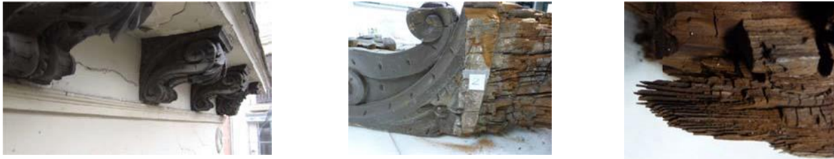
Figure 2: Decorated corbel below the cornice and in the receiving state
